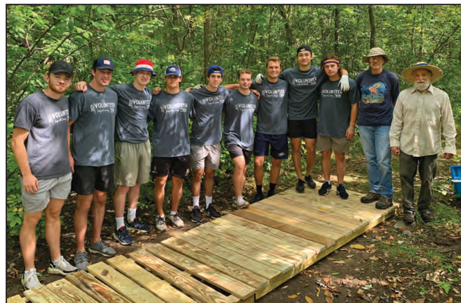
UNITED WAY'S DAYS of Caring brought out these Middlebury College volunteers to help build out the trail system at Rokeby Museum in Ferrisburgh last month.
